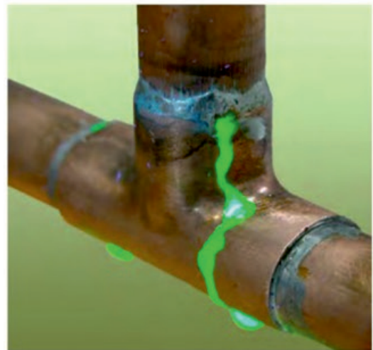
Leak detection in cooling system by use of fluorescent concentrate
